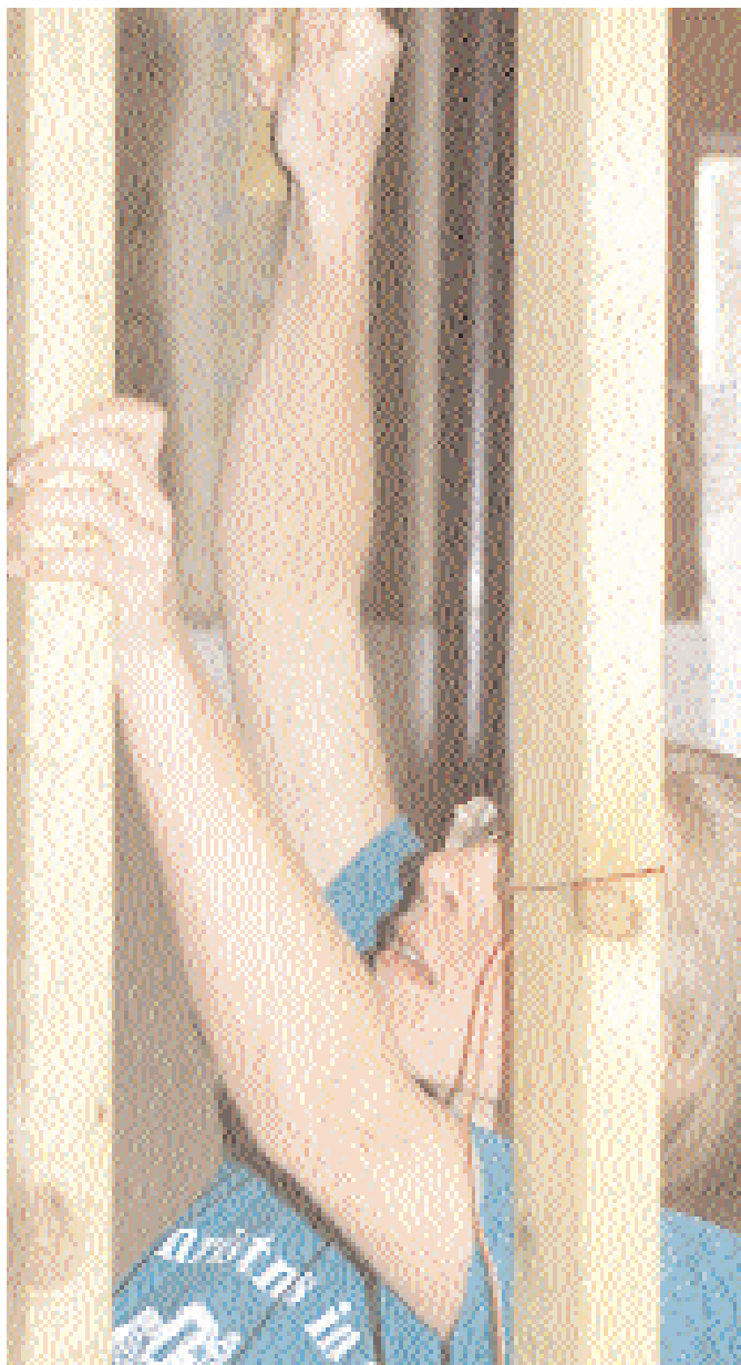
Remodeling and repair tasks accomplished by Peterson volunteers during the "Rebuilding Together with Christmas in April" project also included framing walls in preparation to hang new sheetrock, safety-proofing old trim, prepping new door trim, and hanging new doors.
