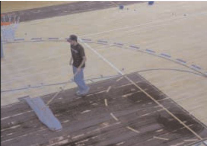
Doug Claes, a construction worker on base, sweeps the floor of gym #2 after it has been stripped. The floor will be repainted and shellacked as will the floor in gym #1.
