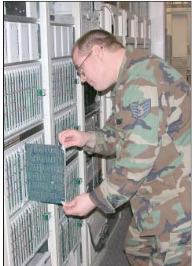
Staff Sgt. David Kisner inserts an interface card into an Integrated Digital Network Service node. The IDNX node is a multiplexer/de-multiplexer used for the cross-country transmission of large amounts of digital data.
