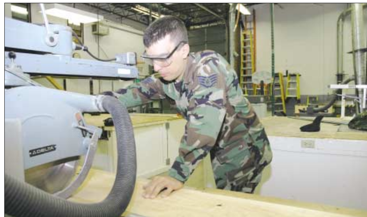
Staff Sgt. David Wilson, structural journeyman, lines up the blade on the radial arm saw before making the cut.
